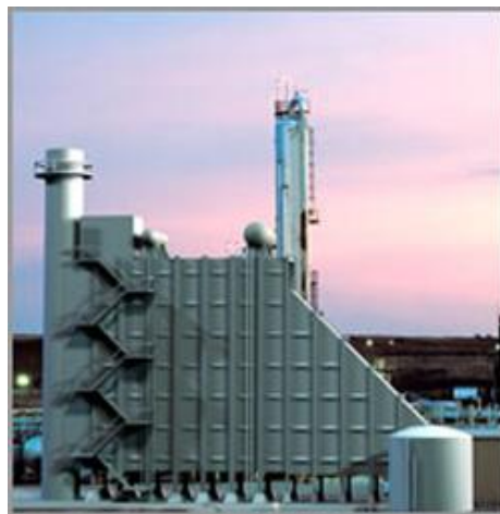
Figure 5.9 Heat Recovery Steam Generator
