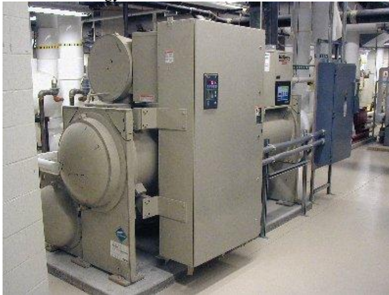
Figure 4.3 High Energy Efficiency Centrifugal Chiller
